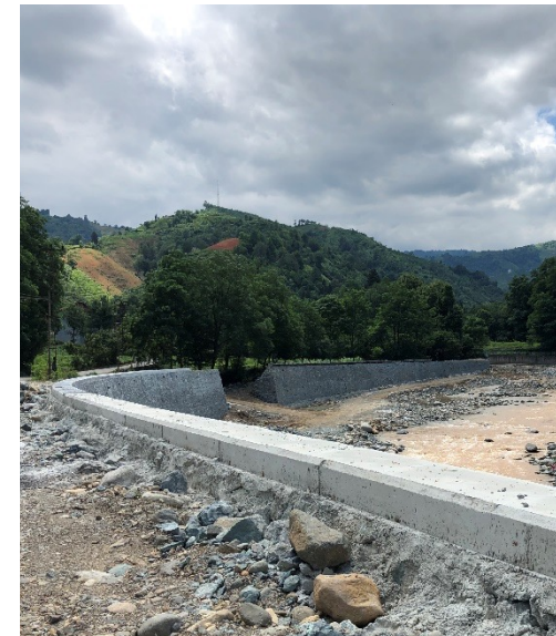
Figure 13 Çağlayan river surrounded by retaining wall which was constructed at the time of second case study trip to Fındıklı, photograph taken by Gül Aktürk, 2019
