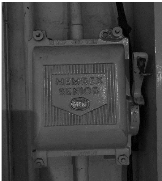
3.6: Standard electrical components installed within Anstruther bunker
