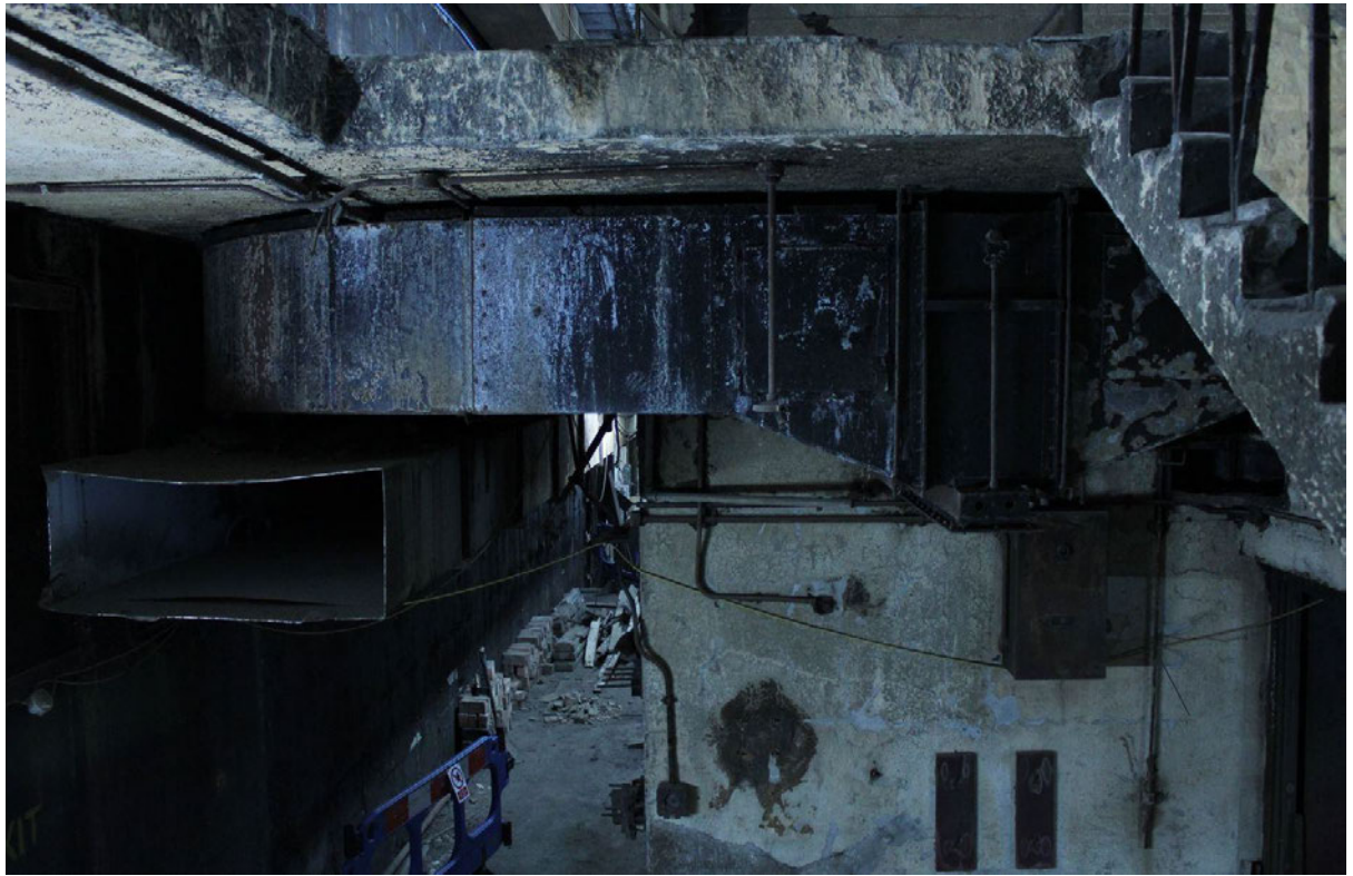
Figure 2.8: Barnton Quarry indicating fire damage and vandalism
