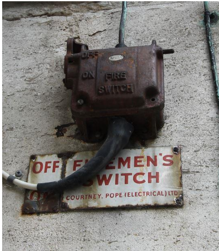
Figure 3.10: Midland Electric Manufacturing Fire-fighting switch located at South Bank
