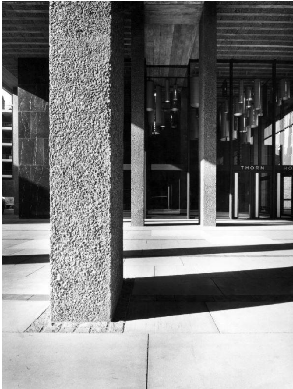
Figure 4.15: Exposed aggregate of in-situ column by washing and brushing, Thorn House, London (RIBApix)
