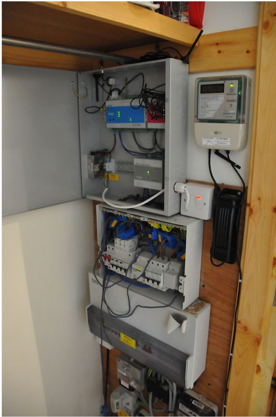
Fig. 1 Data monitoring equipment showing current transformers in the domestic fuse board (centre image) and data transfer equipment (top left) and inline electrical meter (top right). The photo was taken before closing both units
