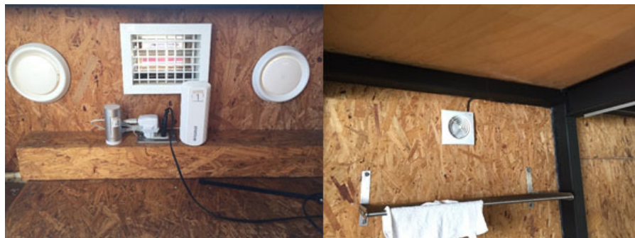
Figure 5: Inlet (A) and extractor fan (B) of the ventilation system at the PH in Mexico City.
