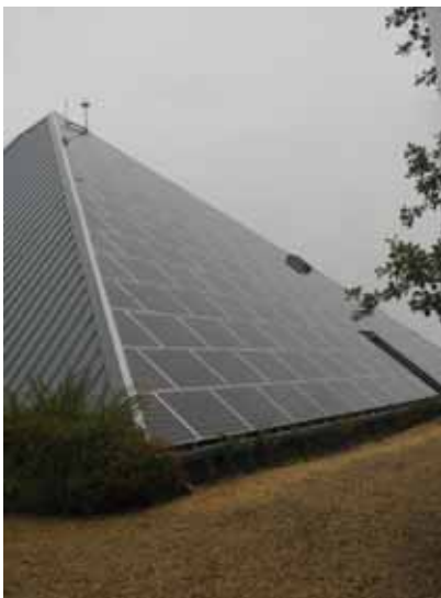
Figure 3: PV clad south facade at Survey Solutions Ltd., Bilston Glen, Loanhead, near Edinburgh – office windows on north and west façade shielded.
