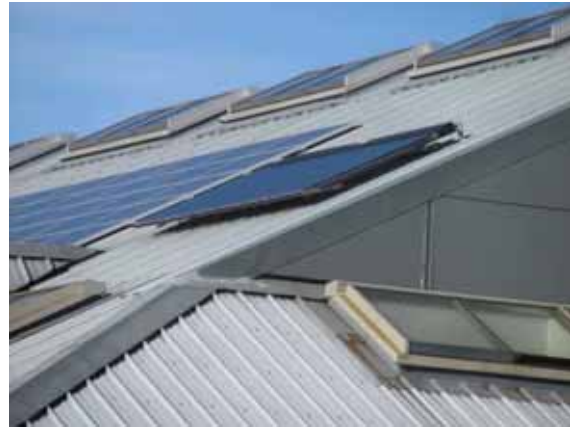
Figure 1b: Roof of new-build community resource, Sporsnis, Ness, Isle of Lewis, indicating building added PV, solar thermal and rooflights.
