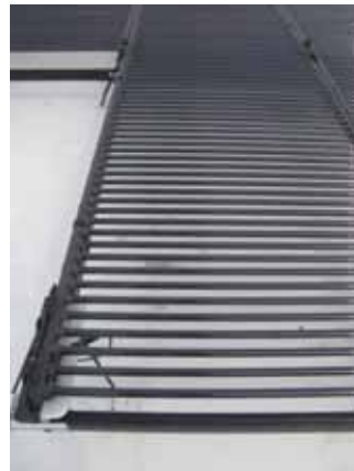
Figure 2b: Solar PV on the roof of Banff and Buchan College, Fraserburgh.
