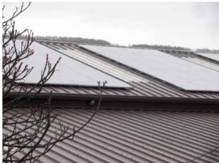
Figure 4: Building added PVs mounted either side of roof lights on roof of Muir Group HQ, Inverkeithing, Fife. Roofscape is visible from the road (position of the photographer).
