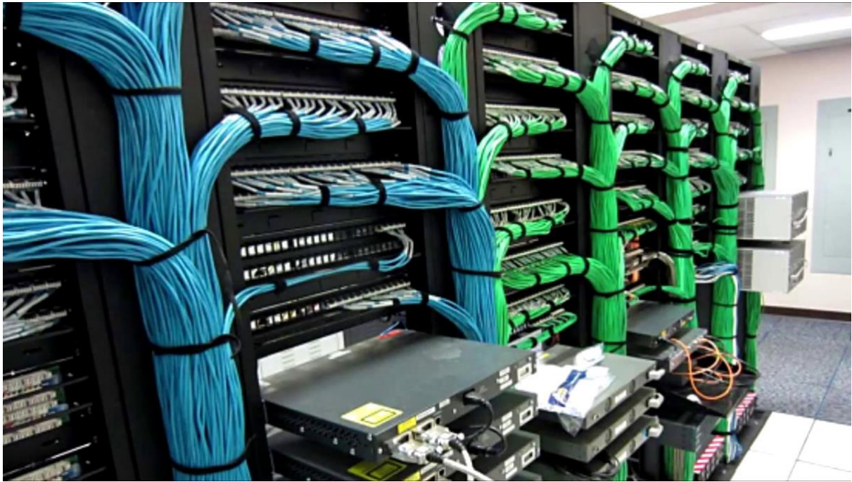
Figure 31 Example of server cable management.
