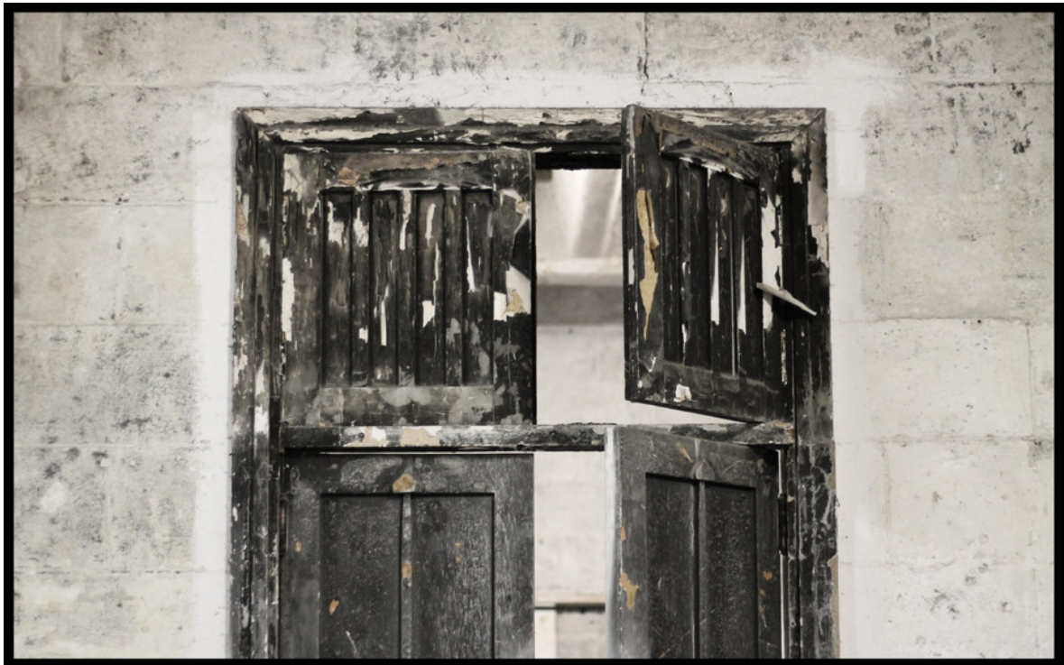
Figure 1. Studio doors of the Mack, left ajar, paint peeling from fire damage. Post fire 1, pre fire 2, February 2018.
