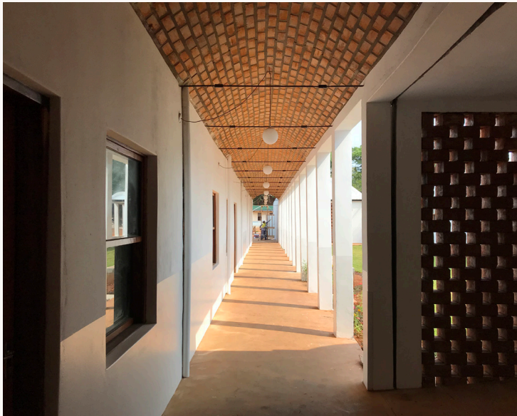
Figure 16. The bottom third of the walls of this hospital are given an extra layer of easy to clean and protective glossy paint. Sachibondu hospital, Zambia, BuildX Studio.
