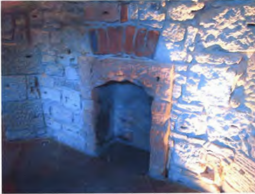
Figure 29 - Inside of the water tank tower at the 3rd floor. The hole of the fireplace is remained. We could know that people stayed this room longer time in this room.
