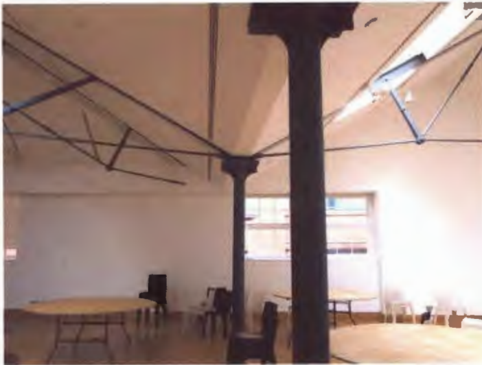
Figure 28 - Current fifth floor. The position of the columns and the inclination of the roof had been changed.
