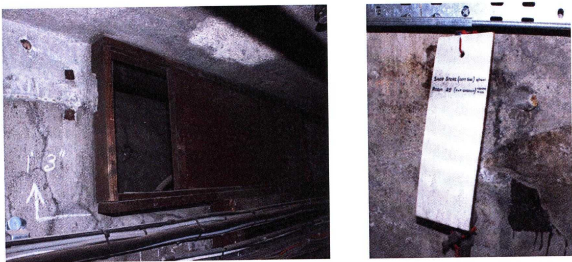
Fig 1.3 Wooden slats that were manually operated allowing clean warm air around the building. Labels indicating corresponding spaces attached to each slat – this example states 'Shop store and room 25.'
