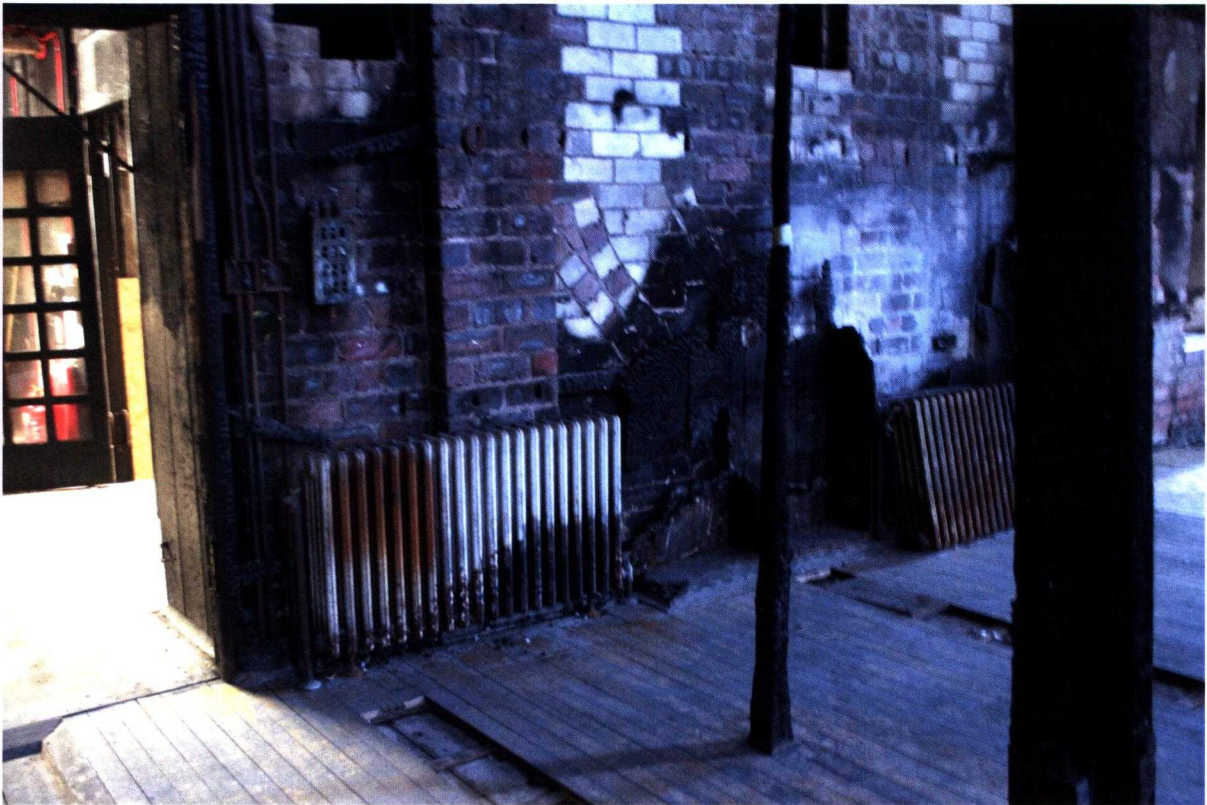
Fig. 4.4 radiators with peeling paint
