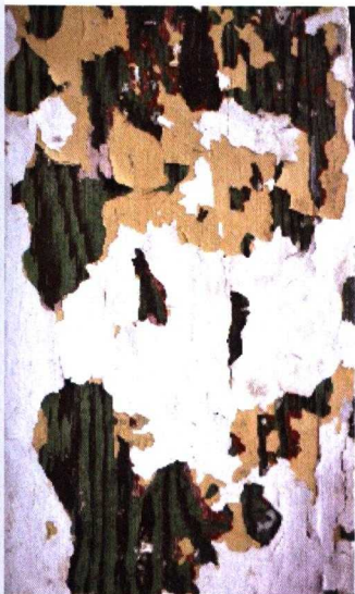
Figure 18. The paint of the interior wall after the fire
