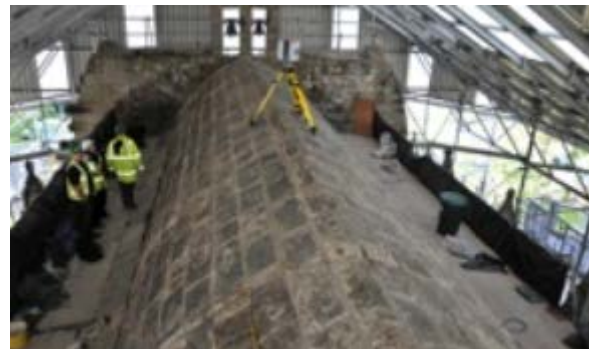
Image Two: Chapel vault with original exterior vault roofing removed and HDS6100 scanner in place
