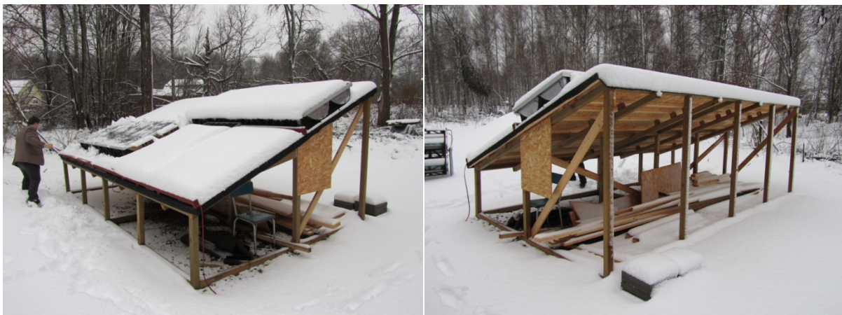
Figure 1: PV/T HR Roof Integrated System Mock-ups Built by Finsun Inresol in Alvkarleby, Sweden
