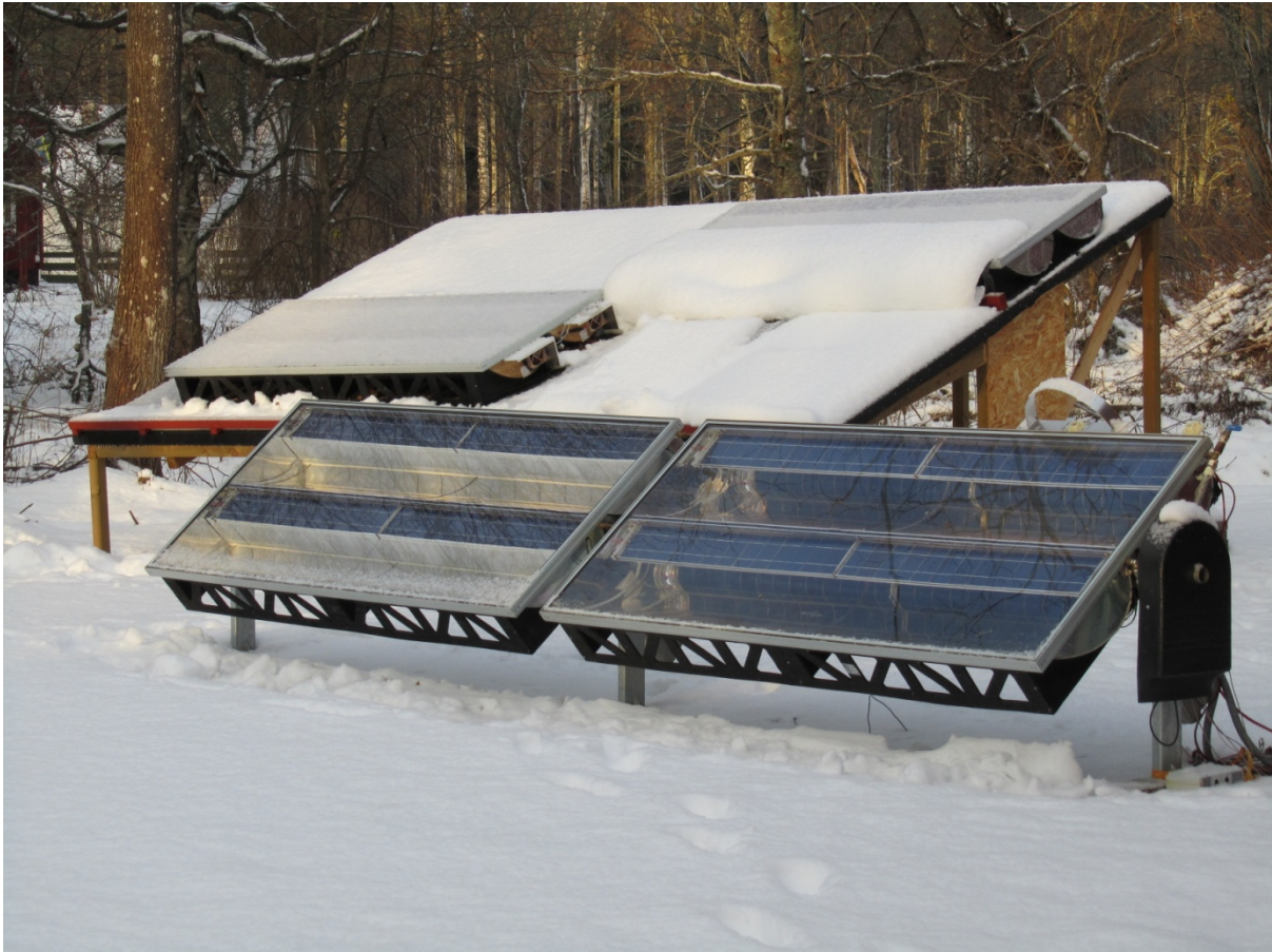
Figure 3: Water-circulated PV/T HR System Mock-up Equipped with Solar Reflectors
