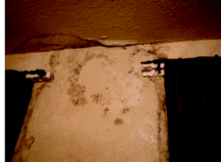
Image 4- Evidence of mould growth within room used for clothes drying in resident's home.
